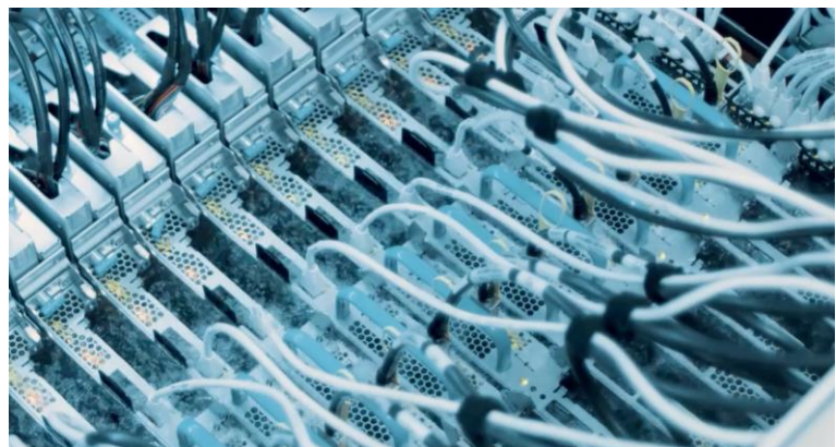
Due to the improved energy efficiency and lower operating costs, immersion cooling has become popular for cooling high-performance computing equipment.
